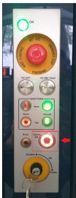
Fig. 8. Safety System control panel with the highlighted Doors OK button.
